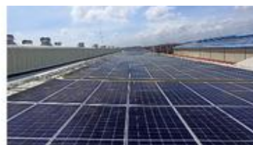
NAMI SOLAR SPEED VINA
